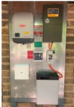
Typical Install, showing solar inverter (top left), battery inverter (top right), Ubi (bottom left) and battery (bottom right)
