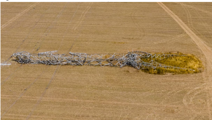
Figure 90. Fallen Victorian 500kV tower
